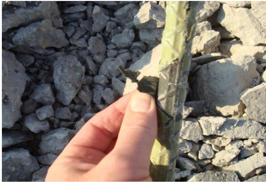
Figure 8: Poor coating adhesion due to inadequate surface preparation of the steel
