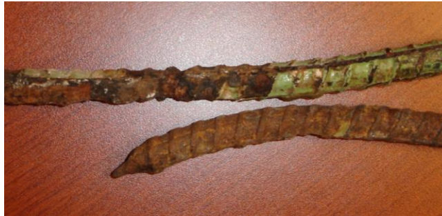
Figure 10: severely corroded bars at longitudinal joint
