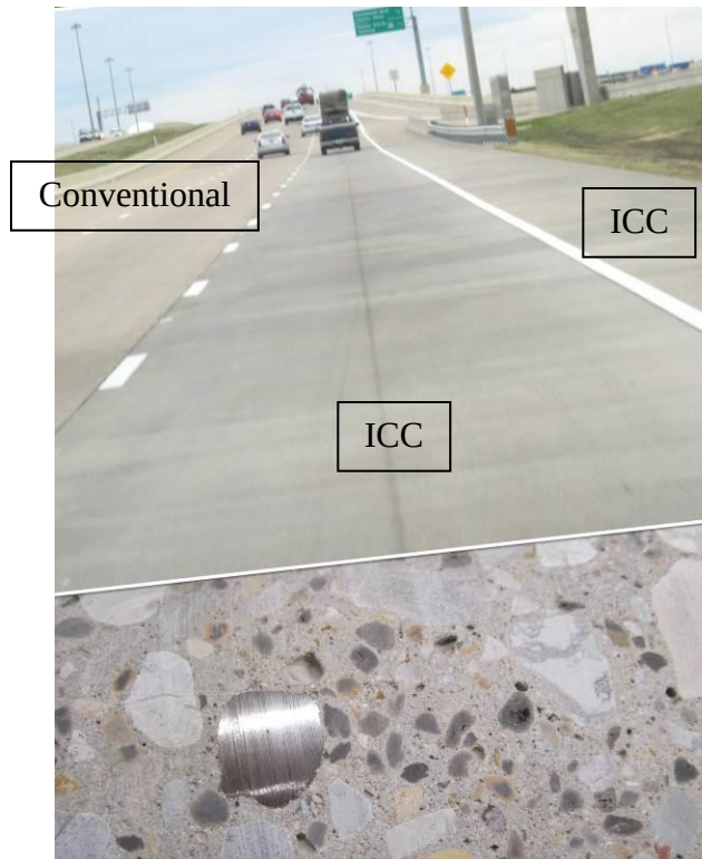
Figure 2. ICC pavement in outer traffic lane and shoulder on Texas SH 121 (top) and view of the core removed from CRCP slab.
