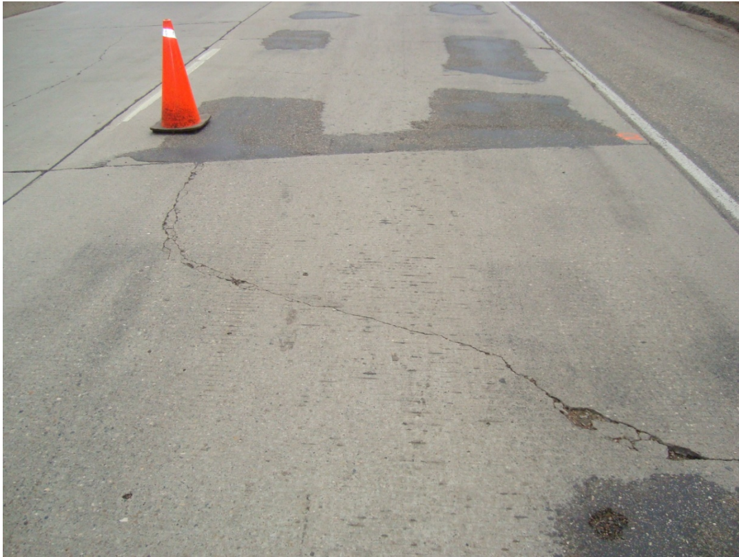
Figure 2. Photo of cracked concrete panel in the outer lane of section 1
