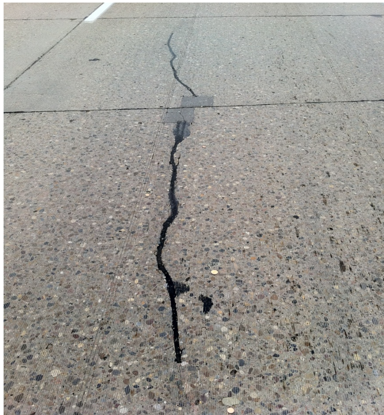
Figure 7. Cross-stitched and spall repaired longitudinal crack
