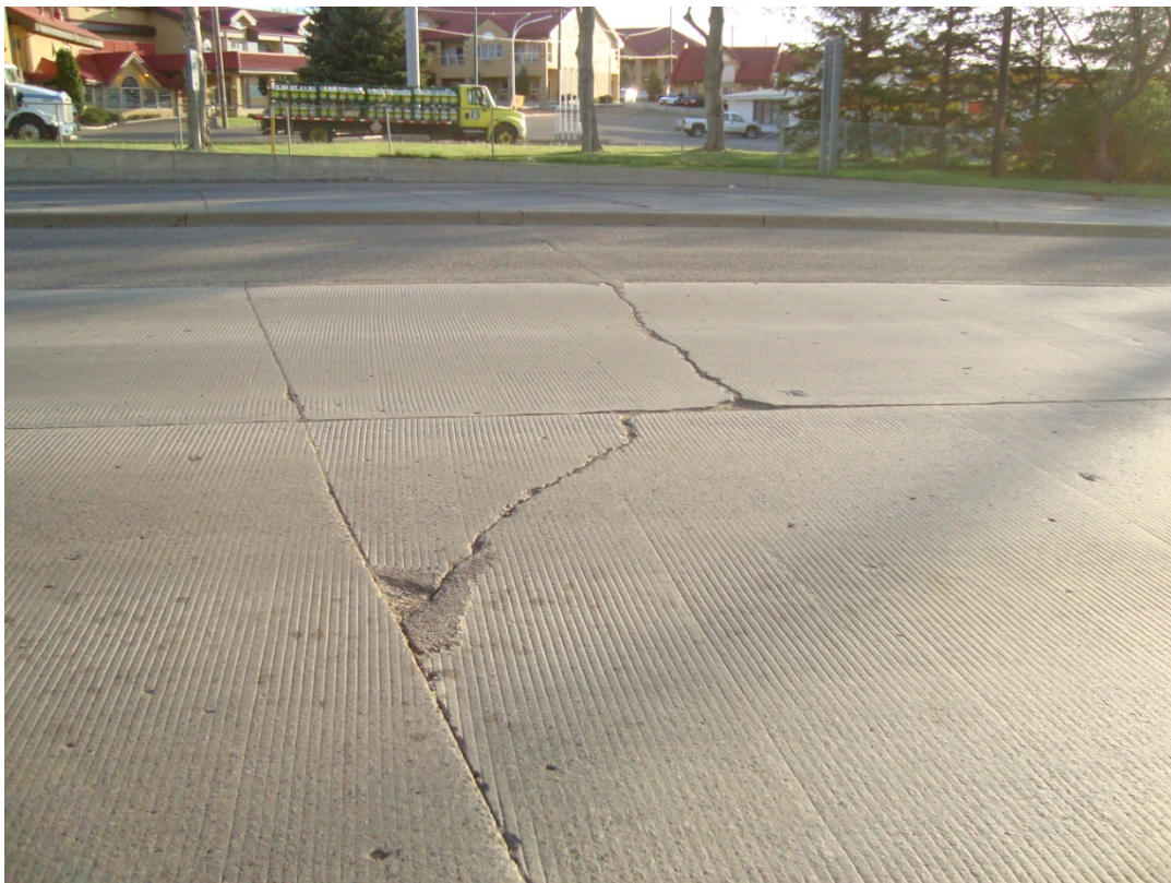
Figure 3. Photo of cracked concrete panels section 3
