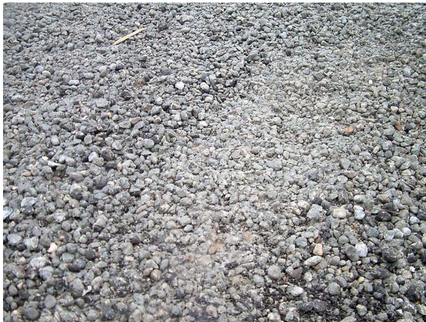
Figure 7. Areas of Severe Raveling
