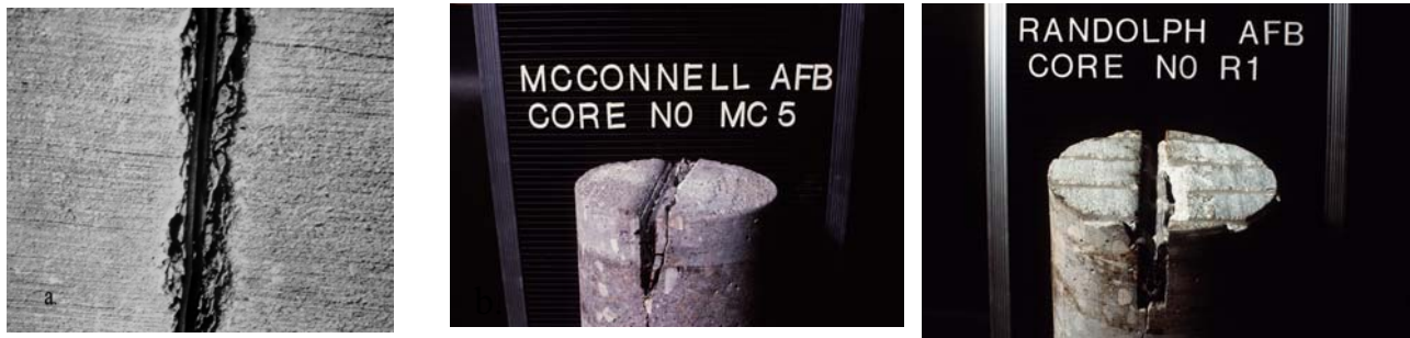
Figure 1. Examples of early-age sliver spalling on joints: (from left to right) a. Grissom AFB, IN freeze-thaw damage due to low entrained air content, b. McConnell AFB, KS freeze-thaw damage due to low entrained air content, and c. Randolph AFB, TX aircraft traffic abrasion and environmental effects damaging a thick covering of weak surface grout with low entrained air and high water-cement ratio.
