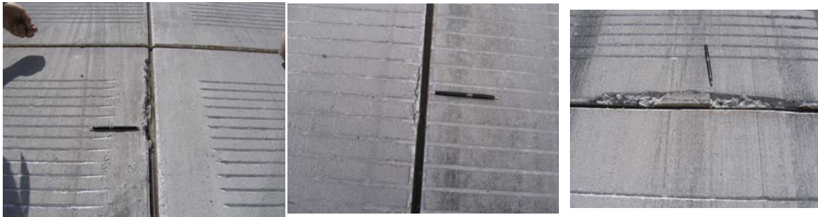
Figure 4. Examples of runway spalling at Airbase A along (from left to right) a. a centerline joint, b. a longitudinal construction joint, and c. a transverse joint.
