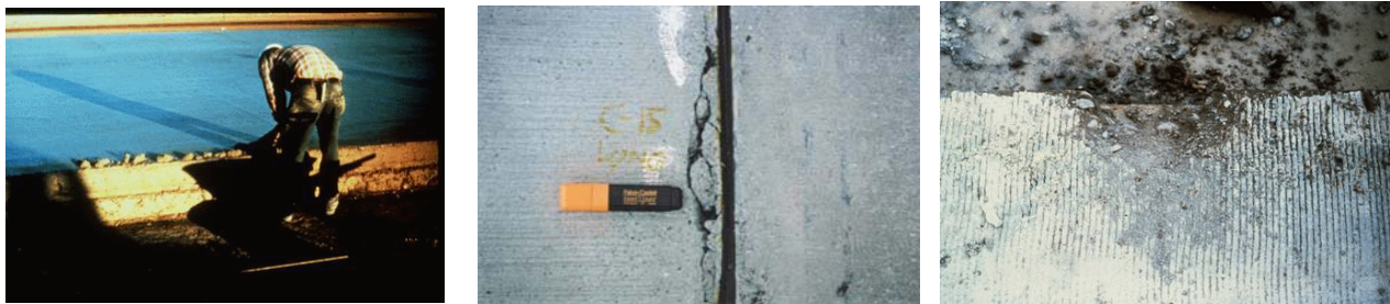
Figure 2. Examples of spalling of edge-slump repairs: (from left to right) a. attempt to repair edge slump using mortar at Travis AFB, CA, b. resulting spalling of these weak edge-slump repairs at Travis AFB, CA, and c. edge-slump repair spalling at Kelly AFB, TX (note original down-slumped surface before repair visible at bottom of spall).
