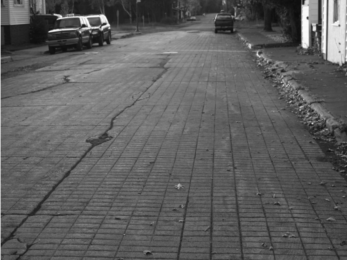
FIGURE 12: Recent picture of Portland Street in Calumet, MI showing no scaling after 100 years of service.
