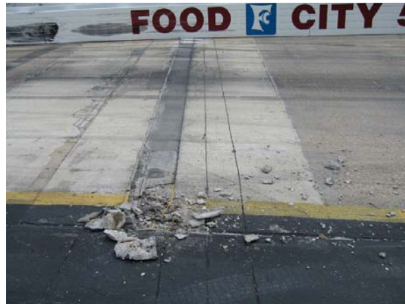
Figure 3 Expansion Joint Failure.
