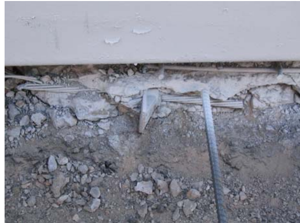
Figure 2 Failed cable anchor.
