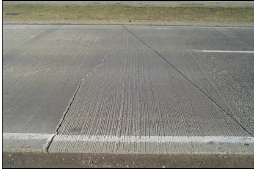
Photo 2. Typical Transverse Crack in Unbonded Concrete Overlay Section
