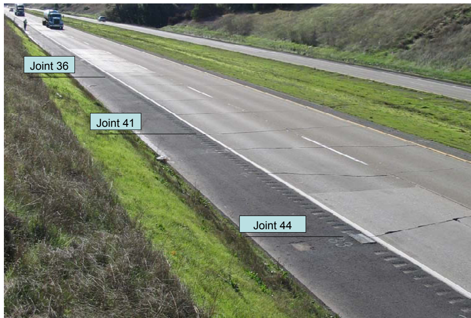
Figure 4. General overview of faulting between Joints 36 and 44 , Ukiah.
