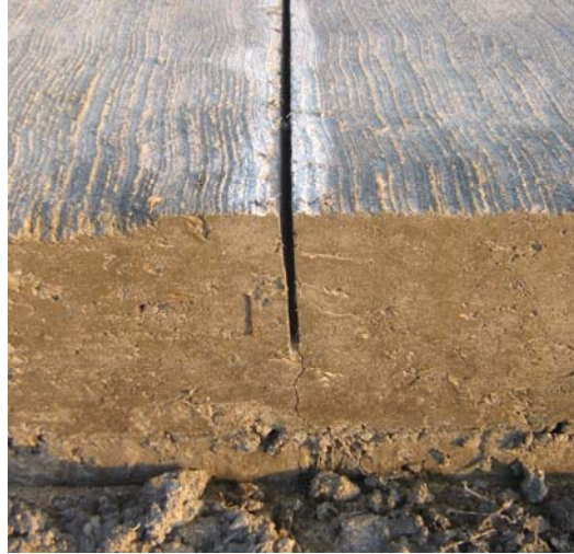
Figure 6 Shrinkage crack formed beneath a transverse shrinkage joint sawn after application of the pavement.
