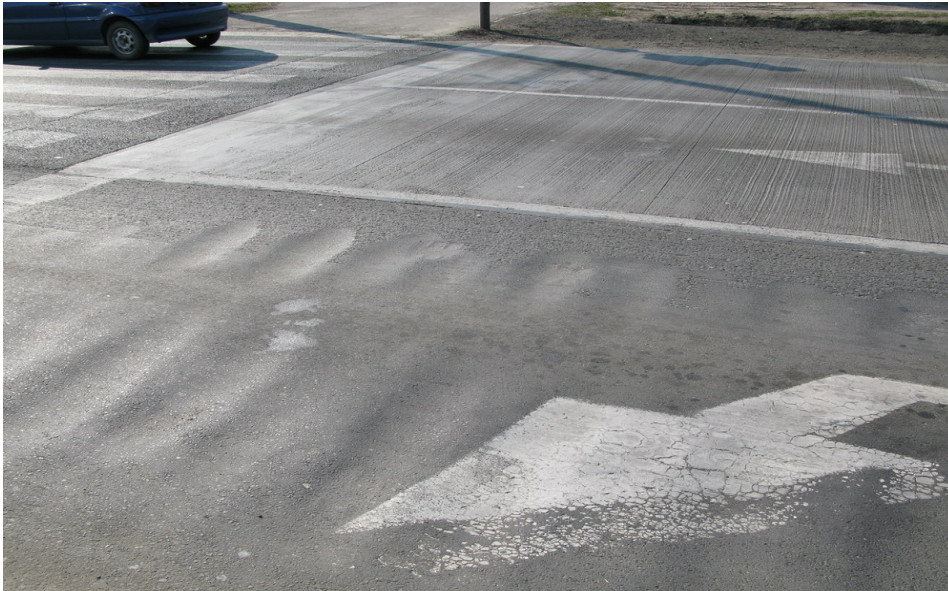
Photo 1 Deformed asphalt pavement surface along the experimental section
