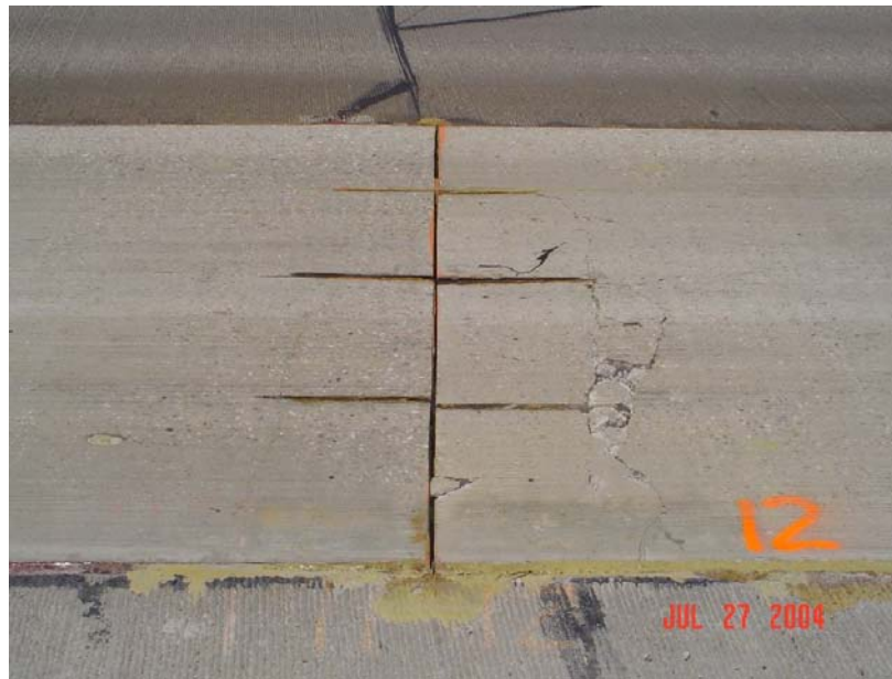
Figure 16 Typical crack patterns
