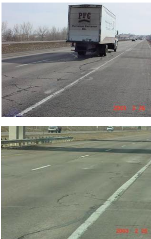
Figure 2. High severity corner breaks with associated spalling.
