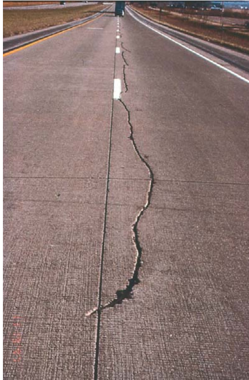
Figure 1. Early Age Longitudinal Cracking
