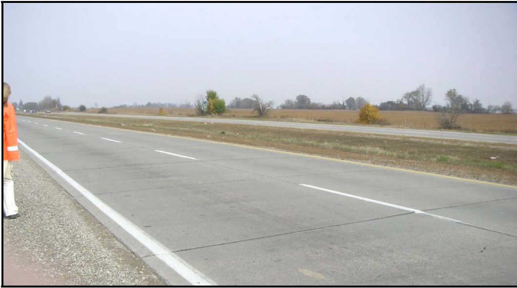
Photo 1. Typical Unbonded Concrete Overlay Condition
