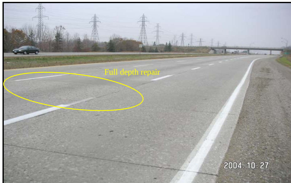
Photo 2. Typical Northbound Lanes Pavement Condition
