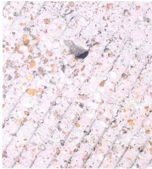
Figure 2 Surface Deterioration of the North 2440 m.
