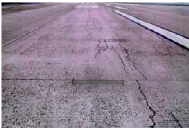
Figure 1 Sample of Cracking Distress in the North 915 m.
