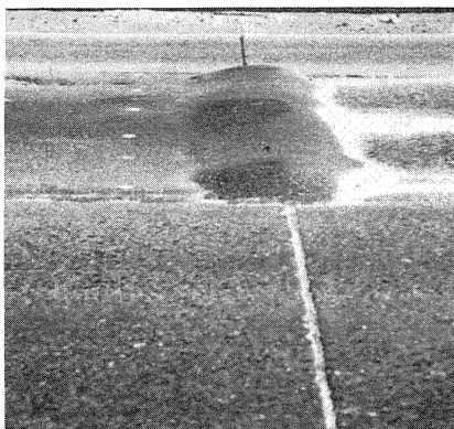
Figure 4. Transverse joint dislocation due to system crushing into the asphalt concrete repair.
