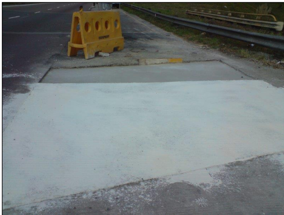
Figure 17: Anchor Beam Jockey Slab (N3/3, km 20.0 Northbound)
