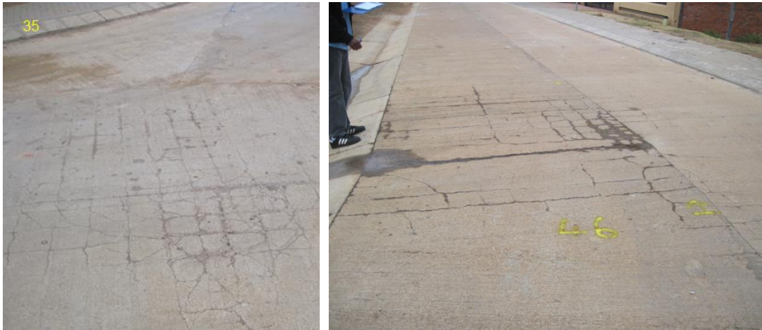
Figure 5: Construction related early failures at the Mamelodi site
