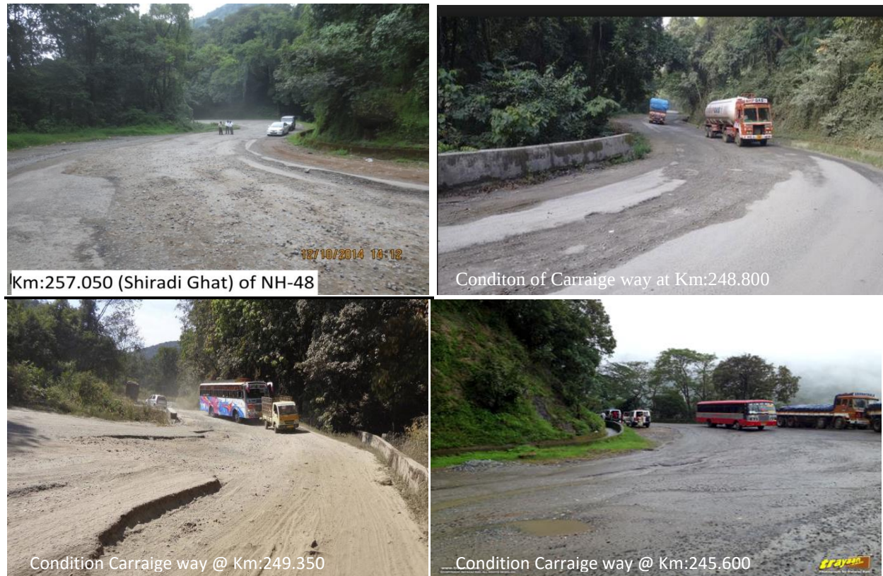
Figure 1 Condition of highway during Rainy season before laying rigid pavement
