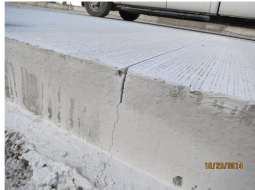
d. Saw cut and resulting crack.
