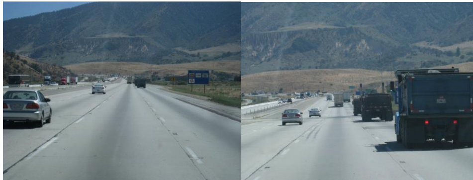
Figure 3. Photo of JPCP project on I-10 in California showing on left no cracks or repairs in outside truck lane, and on right just down the highway extensive cracking and repairs.
