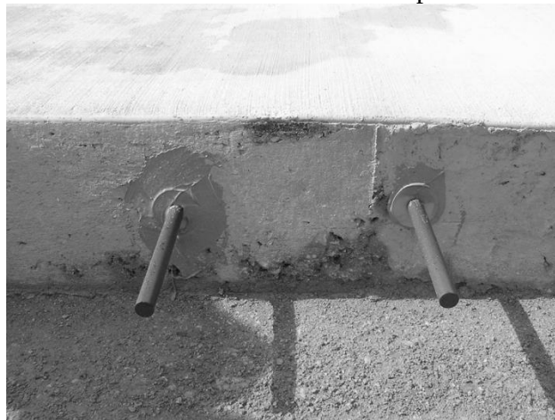
Figure 3. Evidence consolidation issue on an exposed pavement edge.
