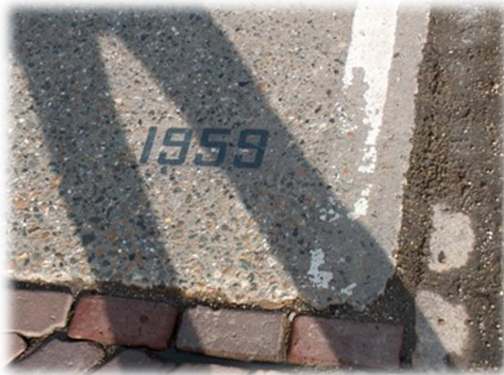
Figure 2: The old concrete pavement on the N625 dates from 1959!
