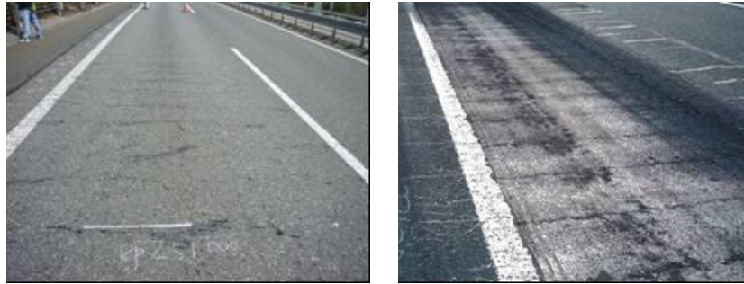
Figure 1. Transverse Cracking on the Asphalt Surface.
