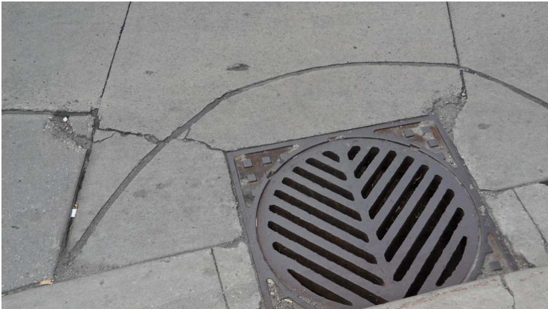
Figure 9. Cracking near catchbasin.
