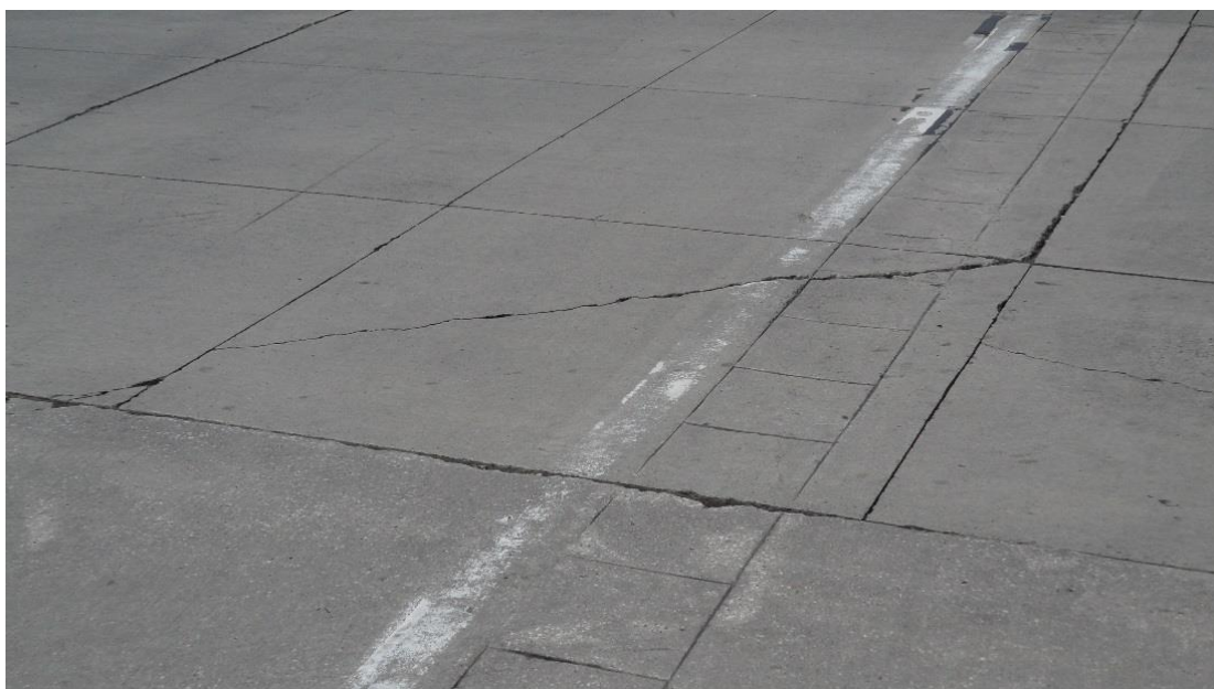
Figure 10. Cracked slabs in crosswalk area.
