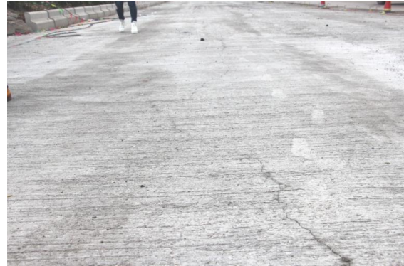
Figure 13. Longitudinal crack at the end of the test section.
