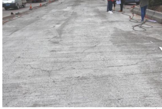
Figure 15. Irregular cracks at the end of the test section.
