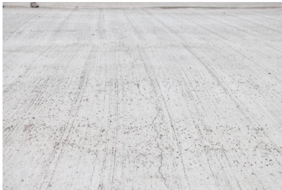
Figure 12. Typical transverse cracks in the CRCP section.
