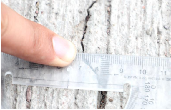
Figure 14. Transverse crack width of initial crack.
