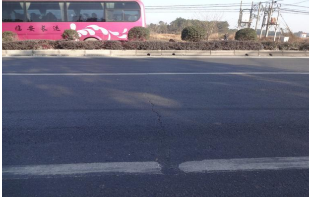
Figure 17. Transverse reflection crack in the HMA.
