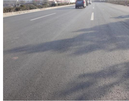
Figure 18. Longitudinal reflection crack in the HMA.
