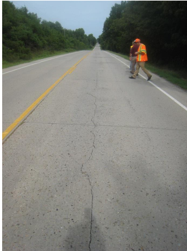
Figure 4. Longitudinal crack in Section 2.
