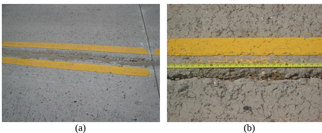
Figure 6. Longitudinal joint deterioration with (a) and without (b) sealant.
