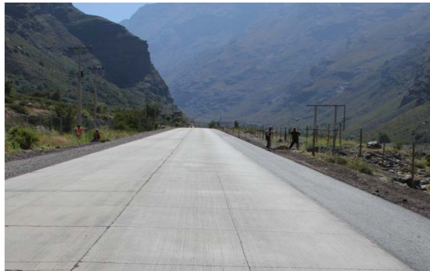
Figure 5. Route 78 2.00m x 1.75 m short slabs in area of high built-in curling
