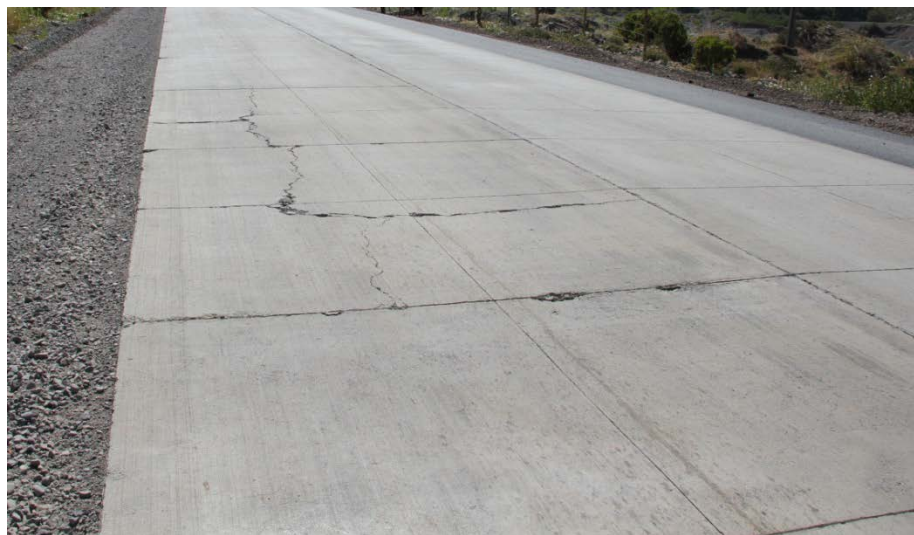
Figure 4. Route 60 - 4 m long by 3.5 wide slab failures designed with AASHTO 1998.
