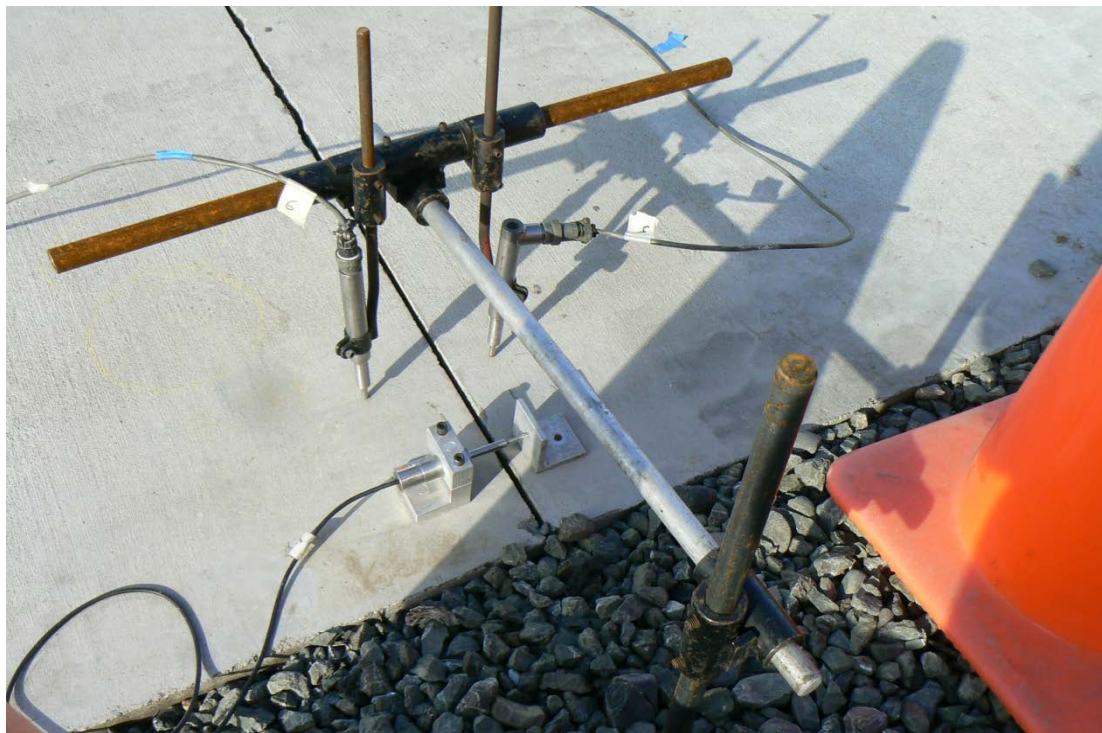
Figure 3: A photo showing the JDMD configuration for monitoring both horizontal and vertical movements at a joint. The horizontal JDMD shown is model DSD800SE5 made by Daytronic, and the vertical JDMDs are model GHSD/GHSDR 750 made by Macro Sensors.
