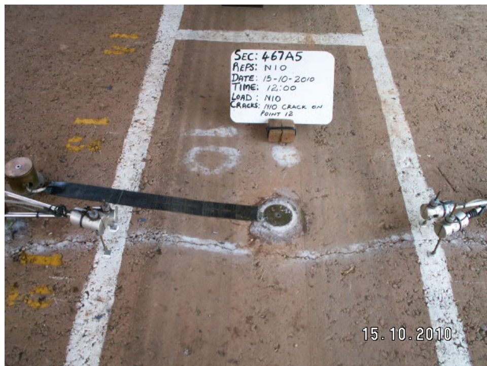
Figure 7: Shrinkage crack at point 12 prior to trafficking
