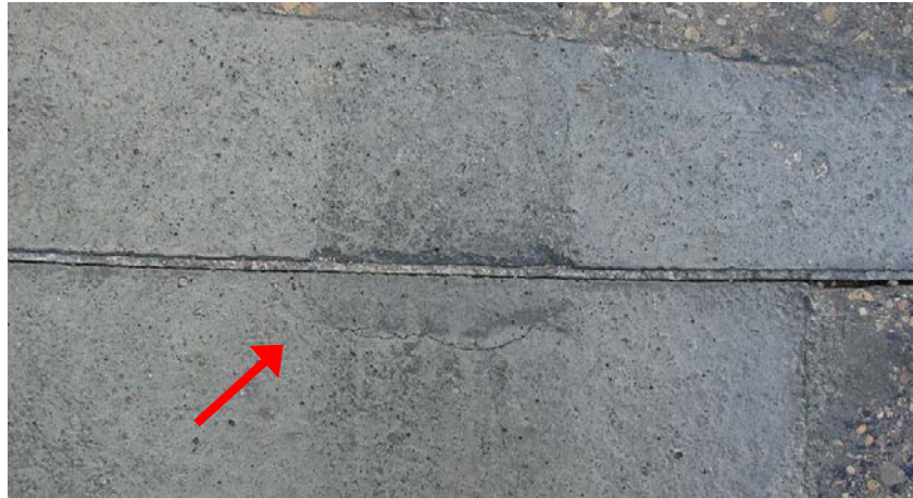
Figure 5: Longitudinal Cracking in the Repair Area
