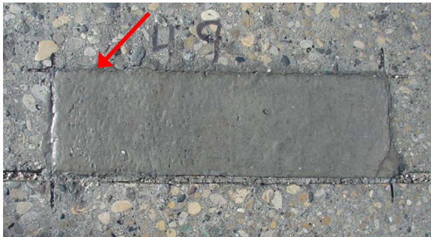
Figure 6: Cracking at the Saw-Cut Surface in the Repair Area
