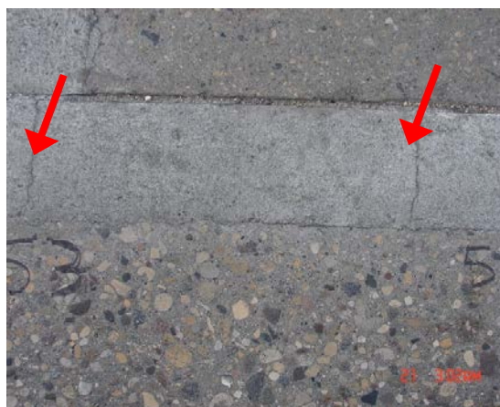
a) Low severity cracking
