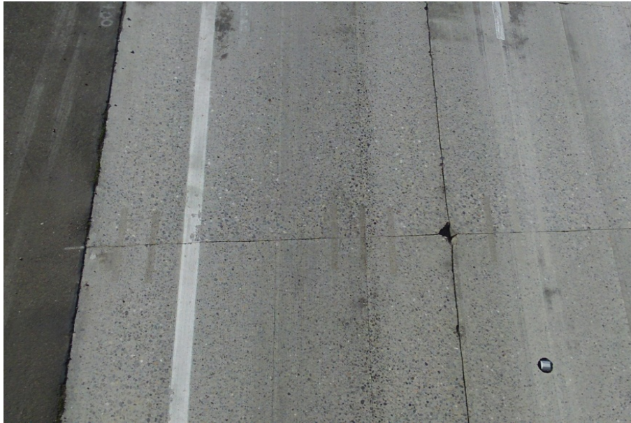
Figure 3. US 50 DBR slots backfilled with polyester polymer concrete seven months after diamond grinding.
