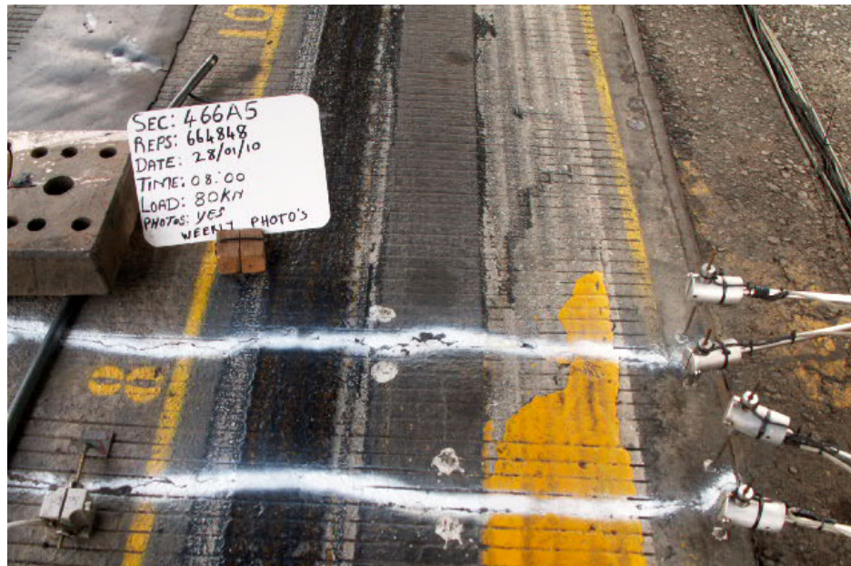
Figure 2: Horizontal and vertical JDMDs and Cracks 3 and 4 after 1.6 million load applications
