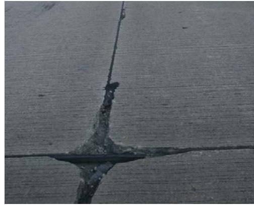
Figure 1. Typical joint deterioration associated with deicer salt scaling (Hansen and Kang 2010)
