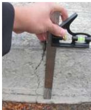
Figure 2b Random crack propagation on the edge of the pavement
