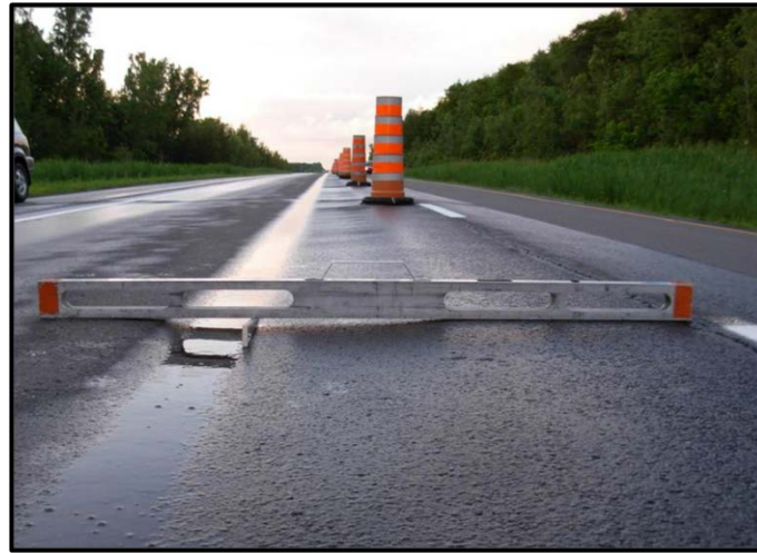
Figure 5 – Condition of Existing Pavement
