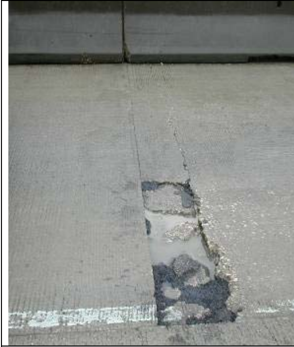
Figure 12-(a) Distress due to improper use of additional rebars
