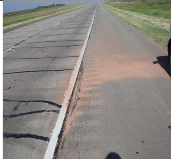
Figure 9-(b) Severe pumping in CRCP with asphalt shoulder
