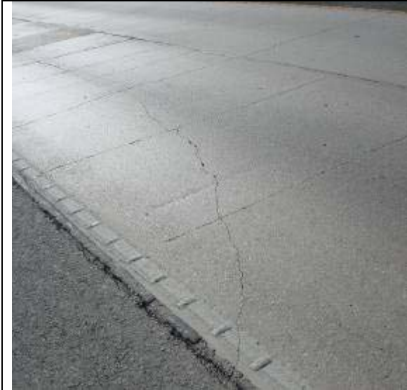
Figure 9-(a) Half moon shape longitudinal crack
