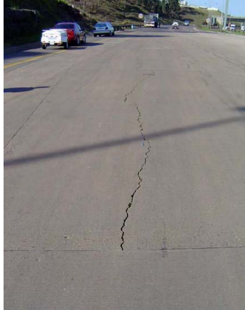
Photo 12: Longitudinal crack in un-doweled jointed concrete pavement
