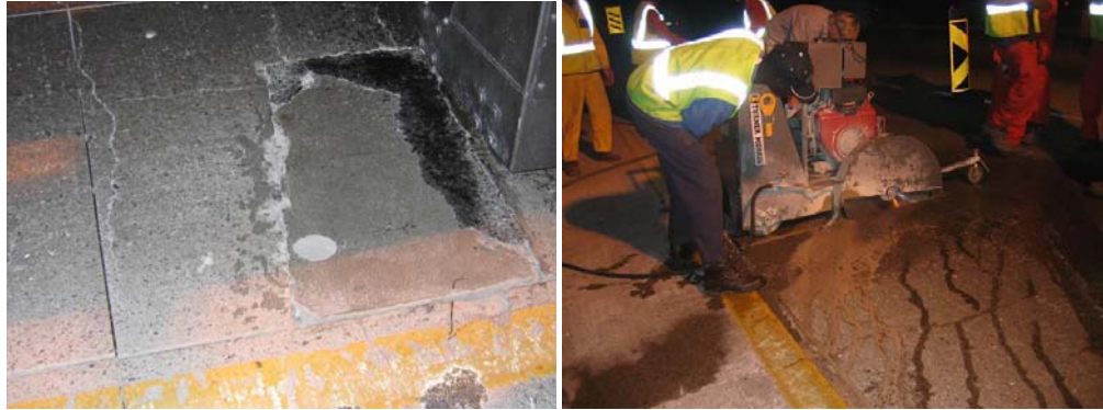
Photo 6: Pop-out in slow lane – temporarily repaired with asphalt (left)
