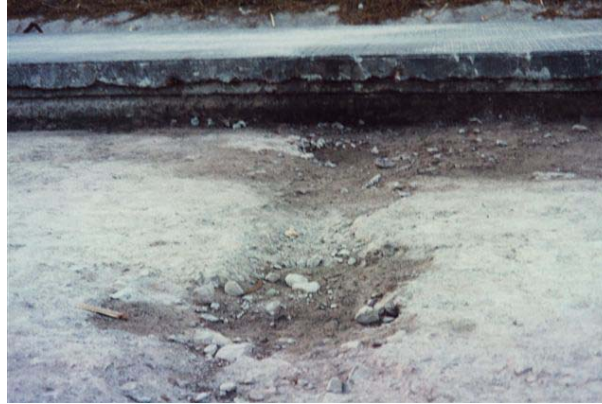
Photo 13: Erosion trenches in subbase beneath transverse and longitudinal joints in concrete pavement
