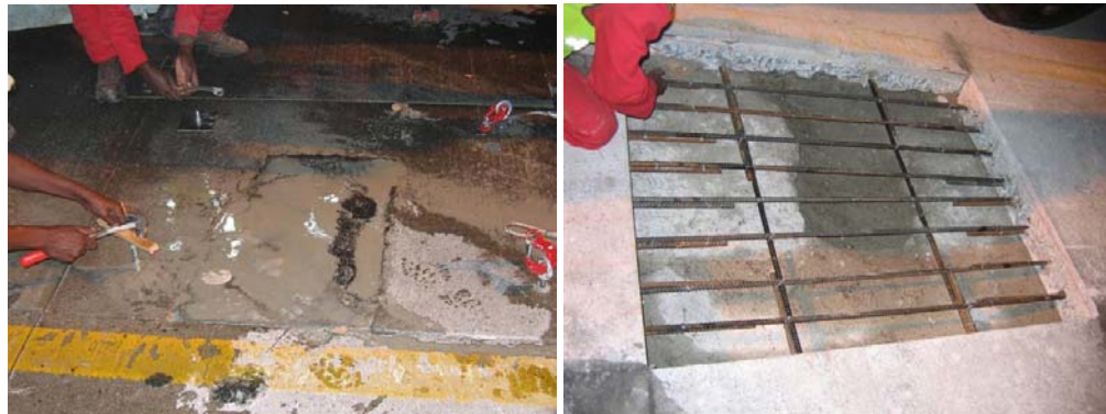
Photo 8: Anchors fixed to lift out failed concrete (left)
