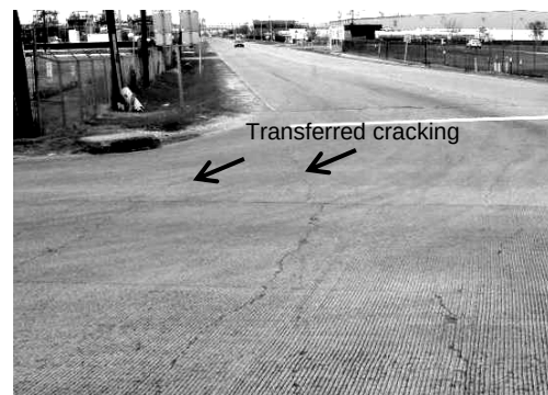
2-b) Transferred Cracking
