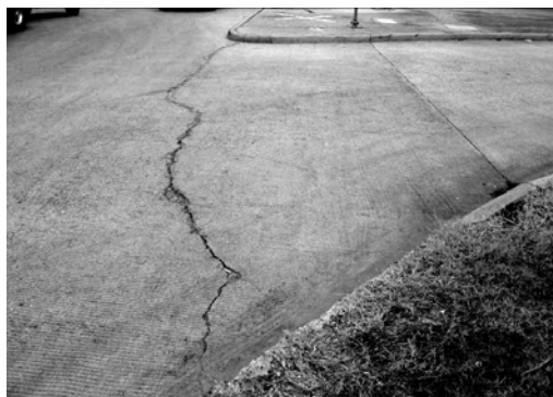
2-c) Uncontrolled Longitudinal Cracking
