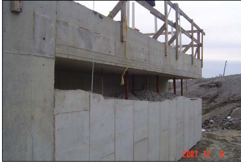
Figure 9 Known void area of concrete filled test shell
