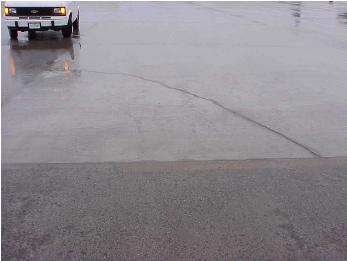
Figure 1. Corner break in concrete overlay due to bond failure at Fairchild AFB.
