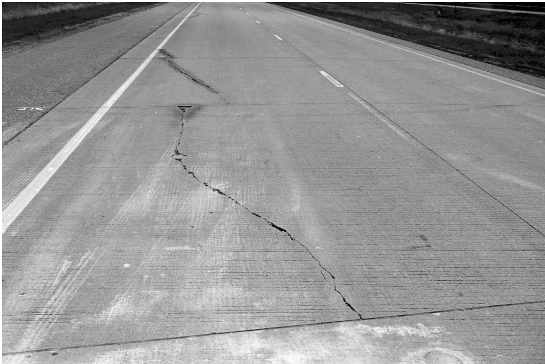
Photo 1. Panel cracking in driving lane of MnROAD test cell 5.
