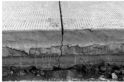
Figure 7. Controlled crack developed underneath the narrow transverse contraction joint at test section S2 established using the early entry dry saw cut method.
