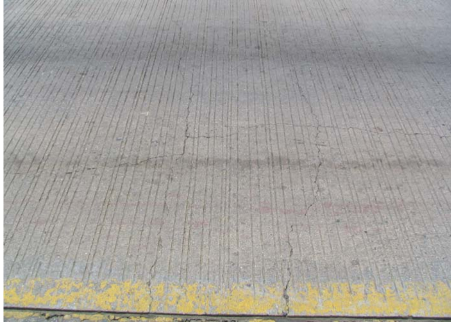
Figure 3. Longitudinal cracks at clustered transverse cracks can lead to punch-outs
