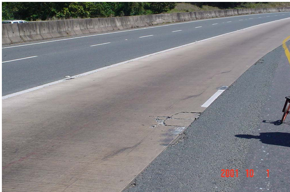
Figure 2. A cluster of cracks, an open edge joint and edge loading lead to a punch-out
