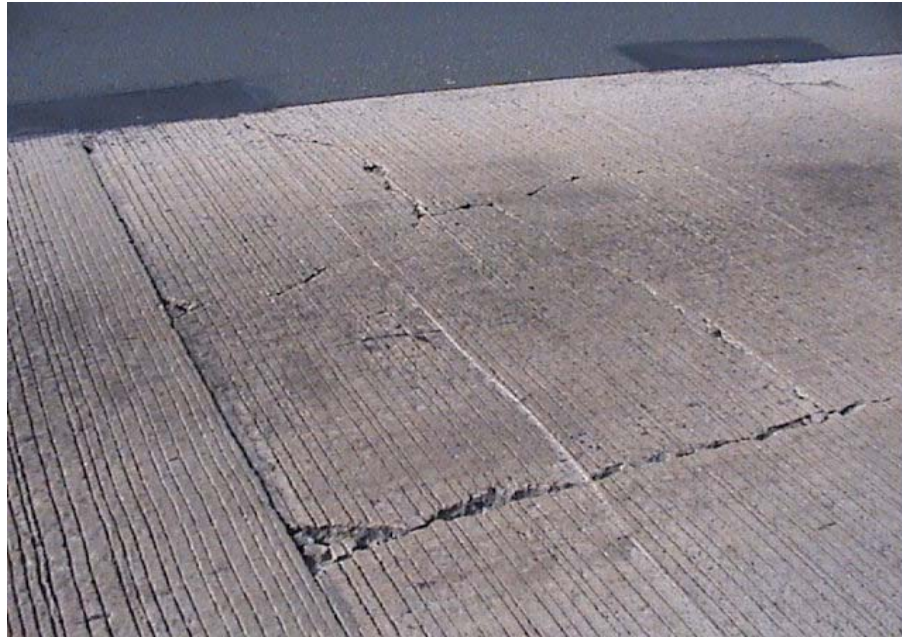
Figure 1. A cluster of cracks at a transverse construction joint and an open edge joint
