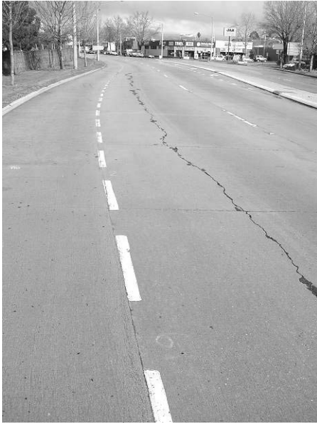
Figure 1.1: Flexural fatigue failure
