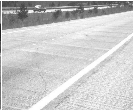
Figure 1.4: Settlement failure (over a skewed box culvert)
