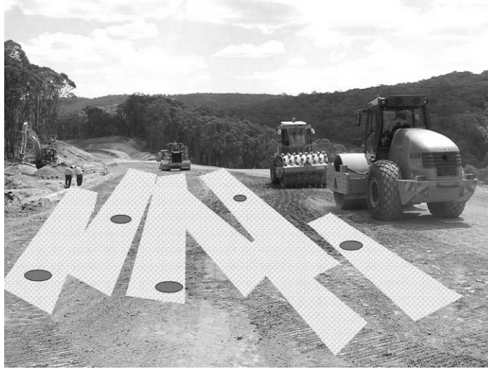
Figure 7. Unsystematic rolling of earthworks
