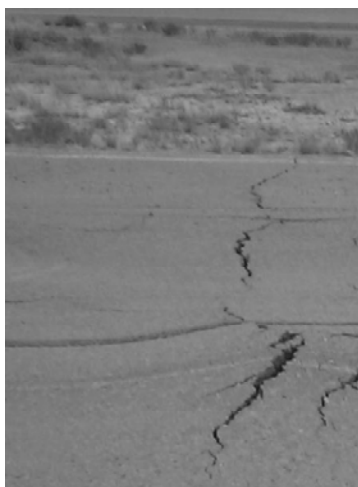
Figure 3. Heaving from sulfate attack on Type V cement-stabilized base, Holloman AFB, NM
