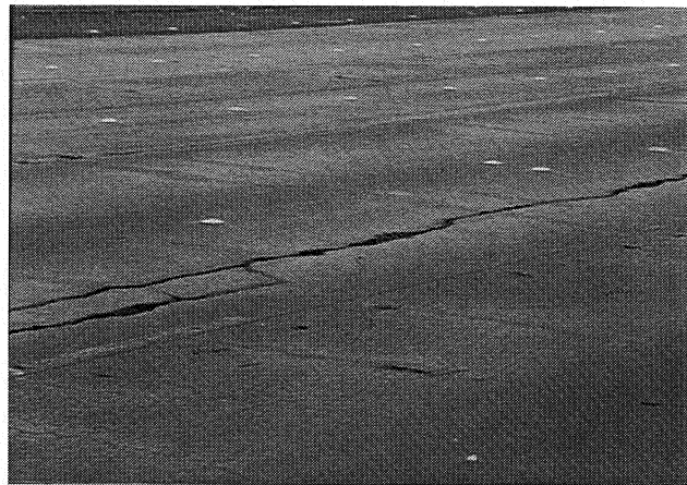
FIGURE 1 Typical uncontrolled longitudinal cracking.
