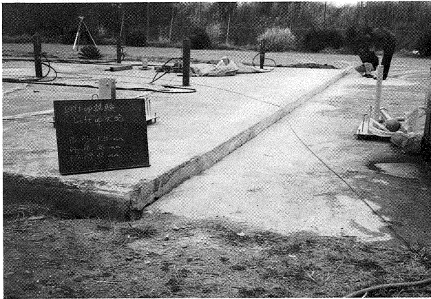
Figure 15. Lifted-up PC slab.
