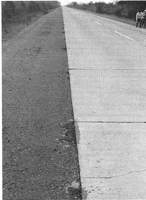
FIGURE 7.- SYSTEMATIC EROSIONS AT LEAVE EDGE CORNERS AND VISIBLE FAULTINGS.
