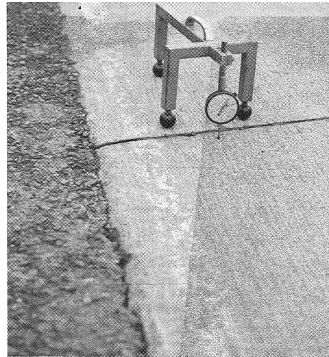
FIGURE 10.- APPARATUS USED FOR THE MEASUREMENTS OF ABSOLUTE FAULTINGS.
