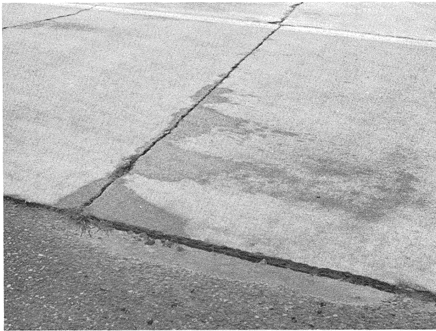
FIGURE 8.- EVIDENCE OF PUMPING AND EROSION AT LEAVE EDGE CORNER IN A 9 - 10 YEAR OLD PAVEMENT.
