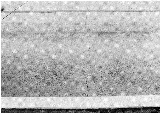
Photo 4 Typical cracks of TBCO on existing CRCP
